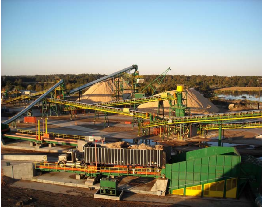
Fulghum Industries provides conveying systems and other heavy duty equipment for the woodyard in Valdosta.
