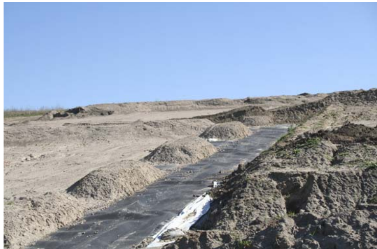
Bunds like this help keep landfill runoff contained so it doesn't contaminate the surrounding area.
