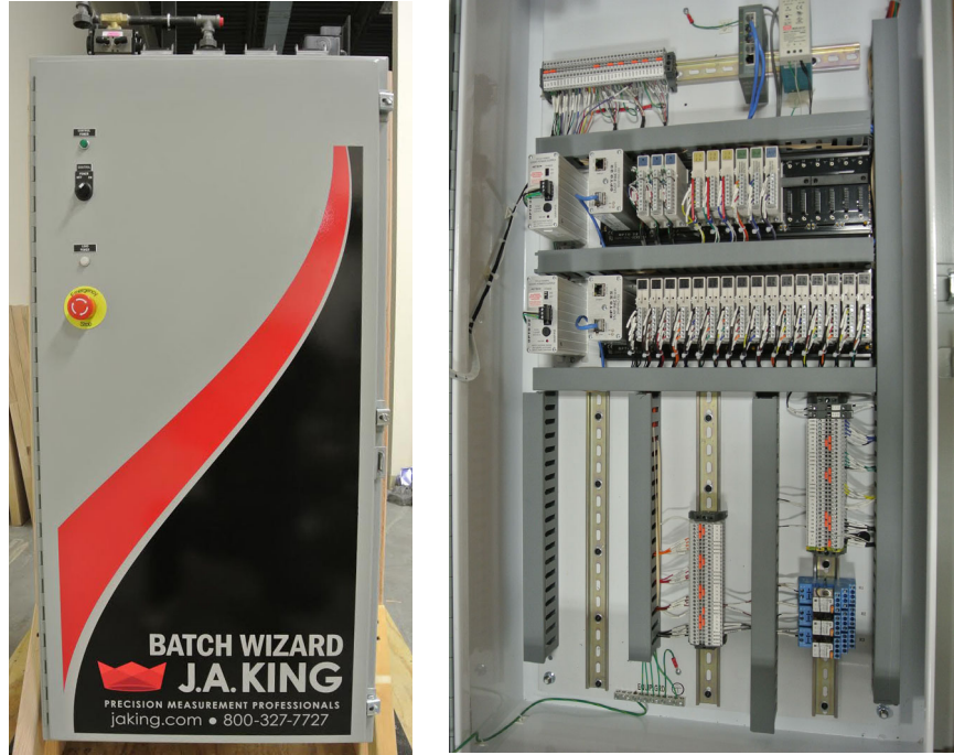
J.A. King I/O cabinet for automated ingredient batching Exterior (left) and interior (right), with Opto 22 Ethernet I/O
