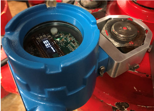
EZ Vision readout and leak detection system
